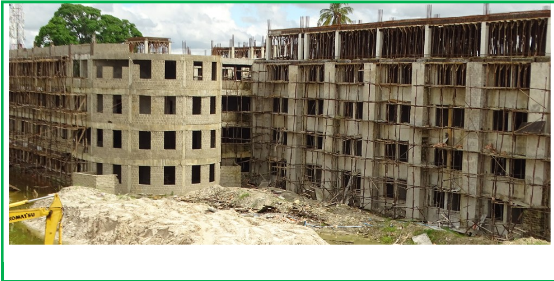
Plate 13: A section of the outstanding construction of a Teaching Hospital at KIUT
